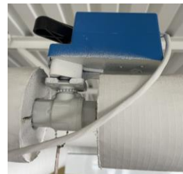
Hot Water Control Valve and Actuator
