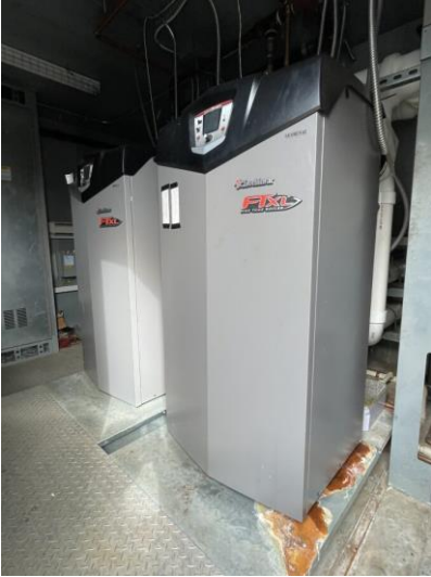
Natural gas-fired boilers
