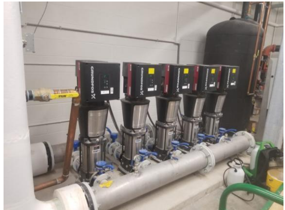
Ground loop pumps
